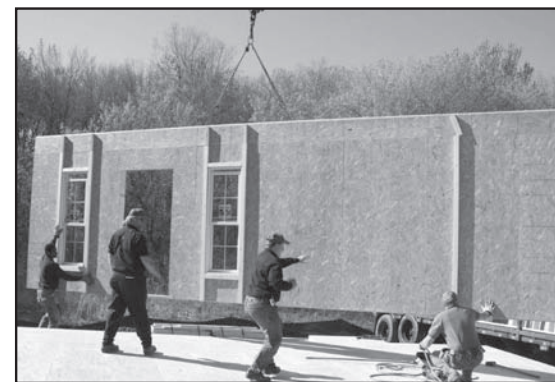
A panel is hoisted into place on a construction site for a panelized home.
